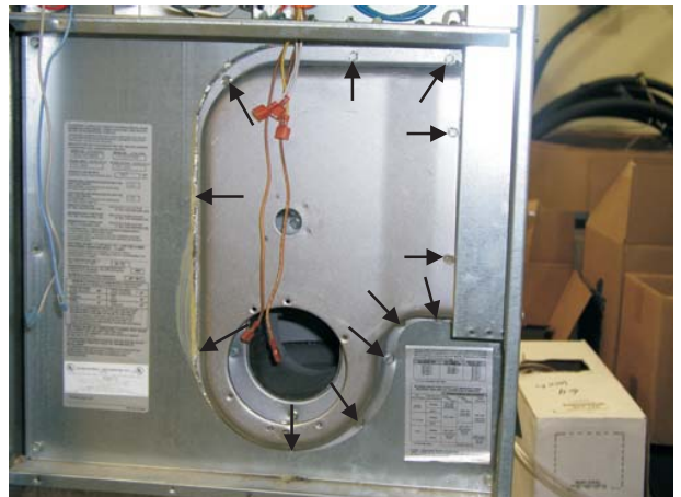
FIGURE 13: Combustion Air Inlet Pan
