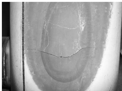
FIGURE 7: Cracked Heat Exchanger
